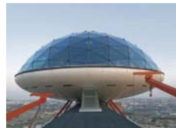
Cúpula del restaurante EVO Hotel Hesperia Tower EVO restaurant's dome Hotel Hesperia Tower Hospitalet de Llobregat 2005
